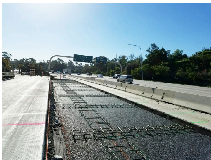
Steel frames provide reinforcement for concrete, which will be poured in the SR 15 median to pave the transit-only lanes.
