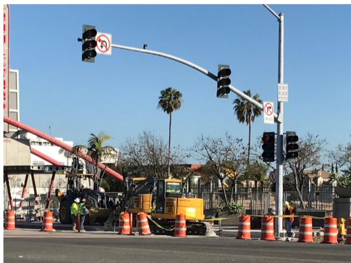
Crews construct upgraded sidewalks along the eastbound side of El Cajon Boulevard at SR 15.
