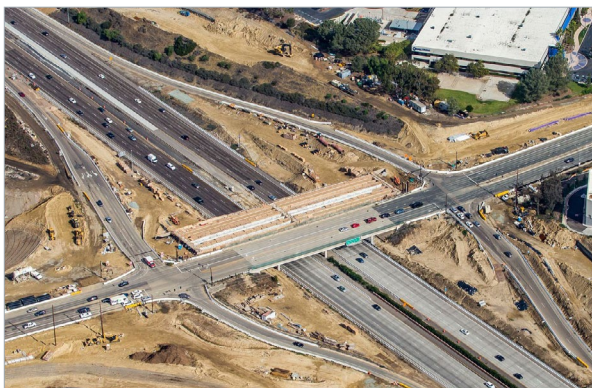
Crews placed utility lines through the new bridge in preparation for the bridge deck concrete pour.
