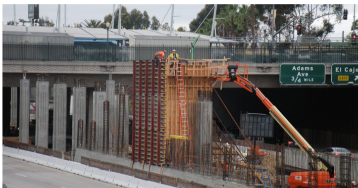
Construction crews work on forming the elevator tower south of University Avenue.
