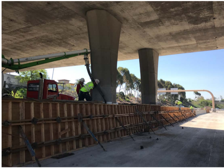
Crews construct a concrete barrier in the SR 15 median south of University Avenue.
