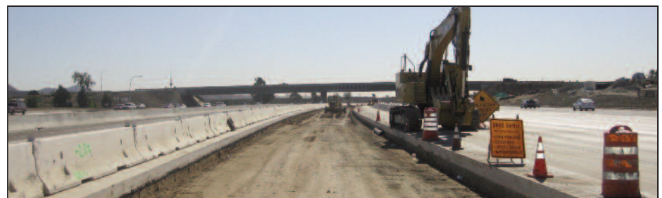
View looking north towards Miramar Way: Construction of the new Express Lanes in the median of the freeway is underway.
