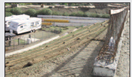
Construction crews placed fiber rolls on a slope near Citracado Parkway to prevent runoff from reaching our local water bodies.
